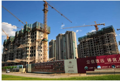
Apartment buildings under construction for a residential project, Beijing, China. Credit: IC Photo via Depositphotos
